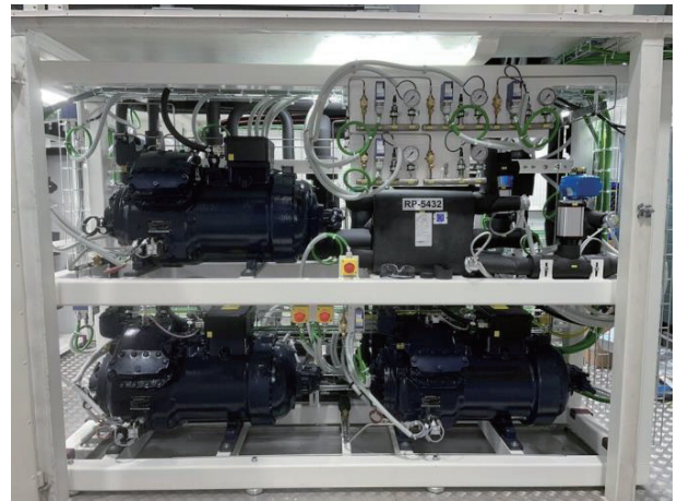
Fig. 6 Photo inside System B container with the two low-pressure compressors installed below the medium-pressure compressor.
